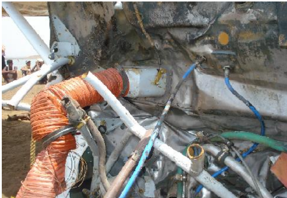
NEW A/C VT-CAI FIRE WALL WITH A/F HRS=708 HRS
